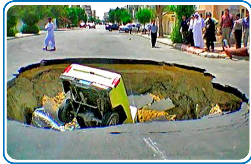
A sinkhole in the middle of a road in Al Khobar City
